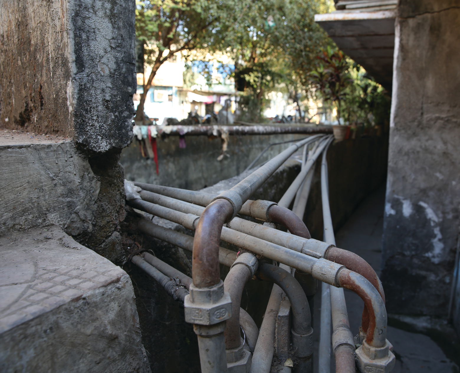
PIPE PUBLICS. A gathering of water service lines in Mumbai. (PHOTO: JESSE SHIPLEY)
