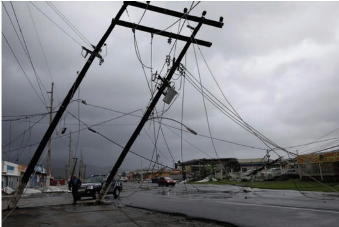
A police officer walks next to damaged electrical installations in Guayama, Puerto Rico. REUTERS/CARLOS GARCIA RAWLINS
